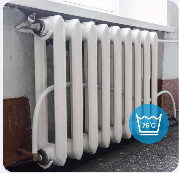
75°C hot water under -10°C ambient temperature
